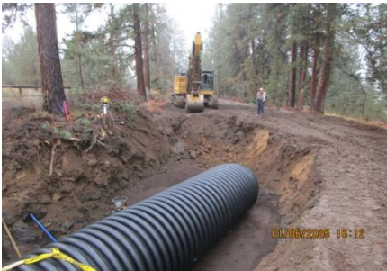
AID MCPH2 - Sta 866+00 54-IN pipe trench excavation + placement pipe bedding material + pipe setting 01-06-25
