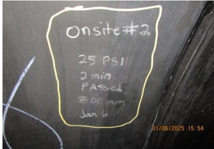
AID MCPH2 - Sta 867+45 POC existing 54-IN pipe, field weld #2, air test results 01-06-25
