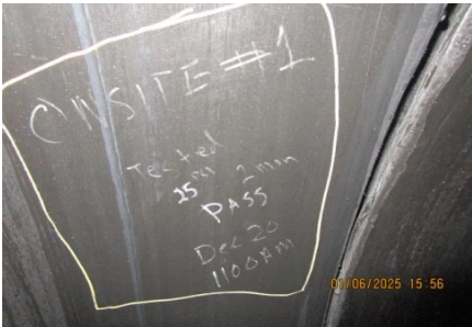
AID MCPH2 - Sta 867+97 POC existing 54-IN pipe, field weld #1, air test results 01-06-25
