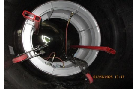
AID MCPH2 - Sta 846+80 54-IN ID profile wall HDPE pipe field joint 25 psi pressure test equipment 01-23-25
