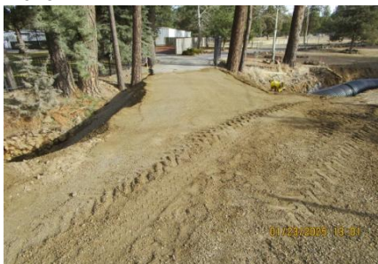
AID MCPH2 Seg2 - Sta. 847+30 54-IN ID profile wall HDPE pipe, Type B Trench backfill (2) 01-23-25
