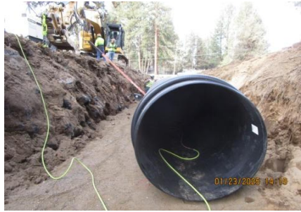
AID MCPH2 - Sta 845+10 54-IN ID profile wall HDPE pipe setting and field joint electrofusion 01-23-25
