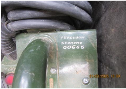
AID MCPH2 Seg2 - Sta. 846+33 54-IN ID profile wall HDPE pipe IntegriFuse Electrofusion Processor Serial 00665 (2) 01-23-25
