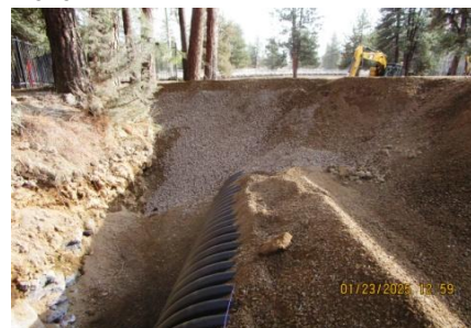
AID MCPH2 Seg2 - Sta. 847+30 54-IN ID profile wall HDPE pipe, Type B Trench backfill (1) 01-23-25
