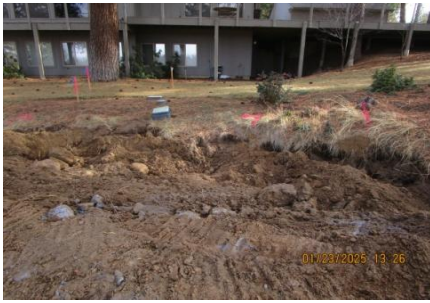
AID MCPH2 Seg2 - Sta. 843+10 + 20 ft - 20 ft pothole for private water and sewer, none found 01-23-25
