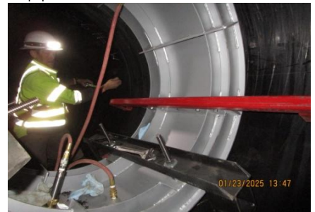
AID MCPH2 - Sta 846+80 54-IN ID profile wall HDPE pipe field joint #61, 25 psi pressure test PASS 01-23-25
