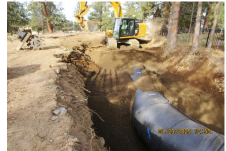
AID MCPH2 Seg2 - Sta. 848+30 54-IN ID profile wall HDPE pipe, pipe zone backfill and compaction 01-23-25
