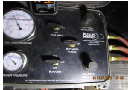
AID MCPH2 - Sta 846+80 54-IN ID profile wall HDPE pipe field joint 25 psi pressure test controller 01-23-25
