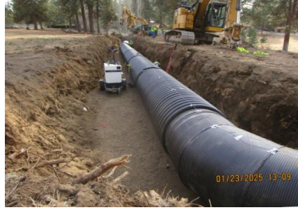
AID MCPH2 Seg2 - Sta. 846+70 54-IN ID profile wall HDPE pipe and fittings install 01-23-25
