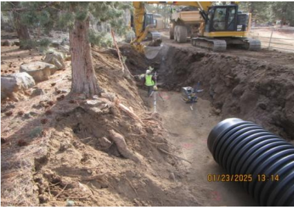
AID MCPH2 Seg2 - Sta. 844+75 trench excavation and bedding 54-IN ID profile wall HDPE pipe 01-23-25
