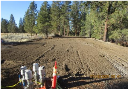
AID MCPH2 - Sta 867+98 54-IN profile wall HDPE Type A trench backfill + rough finish grade 01-16-25
