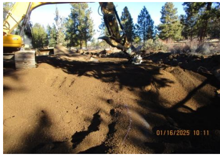
AID MCPH2 - Sta 859+75 54-IN profile wall HDPE Type A trench backfill + compaction 01-16-25
