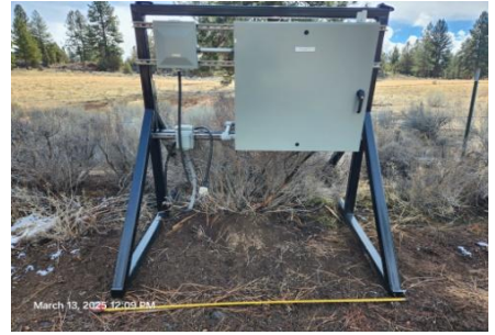
AID MCPH2 - Electrical Equipment Skid 03-13-25
