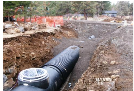
AID MCPH2 - Sta 791+5 54-IN ID profile wall HDPE x 36-IN CO Assly riser + Type B Trench backfill Woodside Rd 03-12-25
