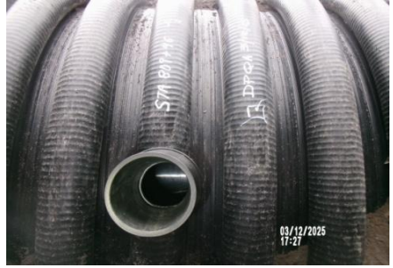
AID MCPH2 - Sta 809+46 4-IN HAS turnout to 1-36152, 2-IN Irrig Service Assly, QA Vis 03-05-25
