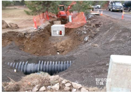
AID MCPH2 - Sta 791+00 54-IN ID profile wall HDPE pipe undercrossing Roats Water and CEC 03-12-25
