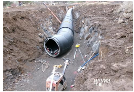
AID MCPH2 - Sta 788+37 54-IN ID profile wall HDPE pipe install and field joint fusion 03-12-25
