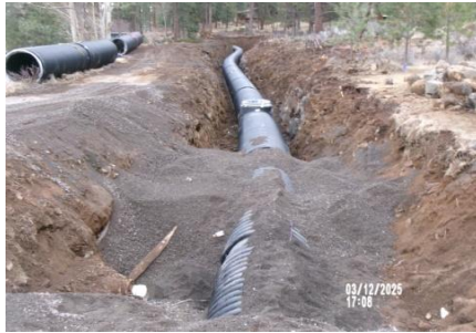
AID MCPH2 - Sta 791+00 54-IN ID profile wall HDPE pipe installed east of Woodside Road 03-12-25
