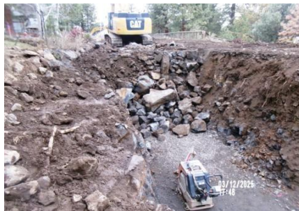
AID MCPH2 - Sta 788+00 54-IN ID profile wall HDPE pipe trench excavation and placement pipe bedding mtrl 03-12-25
