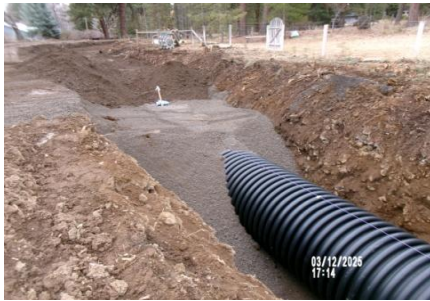
AID MCPH2 - Sta 803+50 54-IN ID profile wall HDPE pipe, initial backfill w toning wire + detect tape 03-05-25
