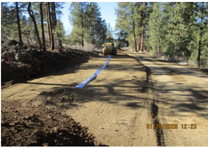
AID MCPH2 Seg2 - Sta. 855+00 54-IN ID profile wall HDPE pipe, Type A trench backfill + detect tape 01-20-25
