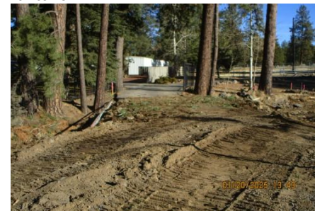
AID MCPH2 Seg2 - Sta. 847+50 existing bridge and abutments removed, temp access provided 01-20-25
