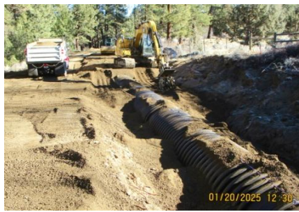
AID MCPH2 Seg2 - Sta. 852+50 54-IN ID profile wall HDPE pipe, pipe zone backfill and compaction 01-20-25
