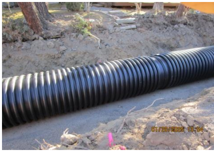
AID MCPH2 Seg2 - Sta. 850+25 private irrigation and electrical, abandoned in place 01-20-25
