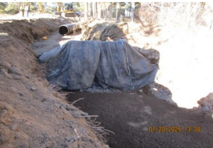
AID MCPH2 Seg2 - Sta. 848+00 existing (2) x 3-IN private water protect-in-place, abandon in place existing irrigation water and power 01-20-25
