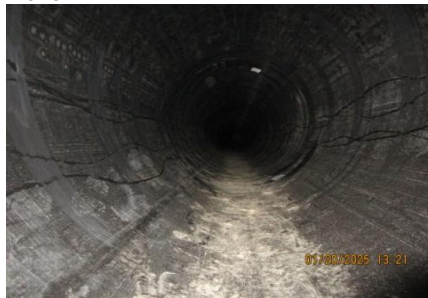
AID MCPH2 - Sta 854+00 54-IN ID profile wall HDPE pipe QA interior after backfill 01-09-25
