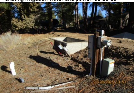
AID MCPH2 Seg2 - Sta. 849+50 irrigation weir box and private electrical, protect in place 01-20-25
