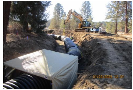
AID MCPH2 - Sta 849+75 54-IN ID profile wall HDPE pipe field joint welding provisions 01-20-25
