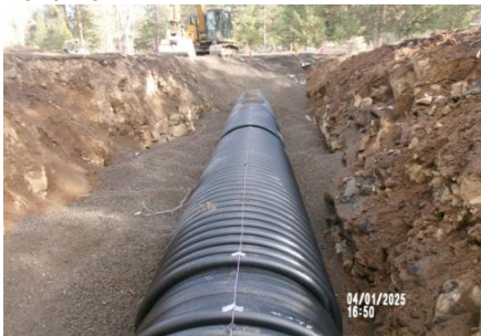
AID MCPH2 - Sta 790+25 54-IN ID profile wall HDPE pipe placement and densification Type A trench backfill (1) 04-01-25
