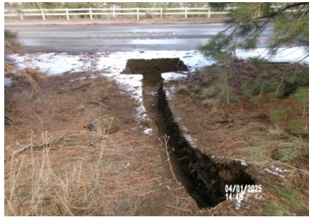
AID MCPH2 Seg2 - Sta. 719+00 existing electrical utility postholed, preparation for installation temp power service Intake Structure 04-01-25
