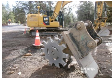
AID MCPH2 - Sta 790+25 54-IN ID profile wall HDPE pipe placement and densification Type A trench backfill (2) 04-01-25
