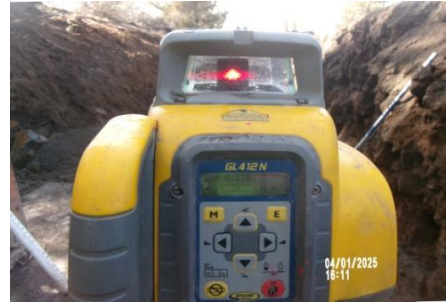
AID MCPH2 - Sta 768+00 54-IN ID profile wall HDPE pipe, placement pipe bedding mtrl 04-01-25
