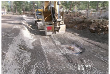
AID MCPH2 - Sta 791+50 54-IN ID profile wall HDPE pipe, 0.75-IN - 0 Aggregate Type A trench backfill in pipe zone 04-01-25
