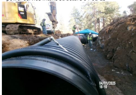
AID MCPH2 - Sta 769+25 54-IN ID profile wall HDPE pipe, installation and field joint fusion 04-01-25
