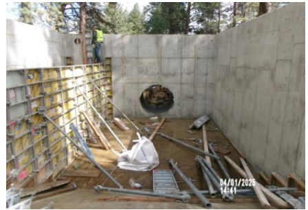
AID MCPH2 Seg2 - Sta. 718+00 Intake Structure, wall form removal, 60-IN ID pipe inlet 04-01-25
