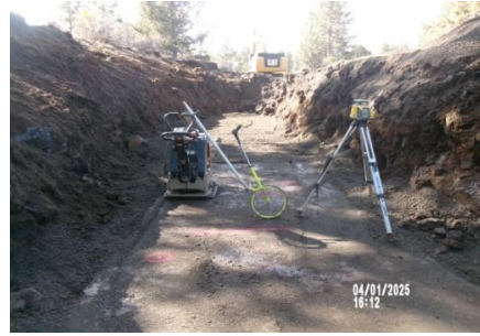
AID MCPH2 - Sta 767+50 54-IN ID profile wall HDPE pipe trench excavation and placement pipe bedding mtrl 04-01-25
