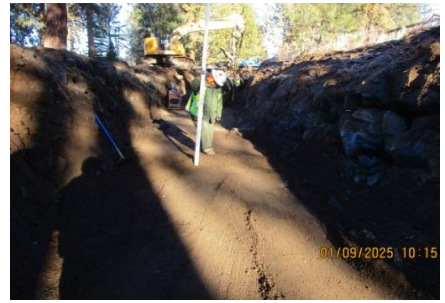
AID MCPH2 - Sta 862+00 54-IN profile wall HDPE pipe trench grade checking pipe bed 01-09-25
