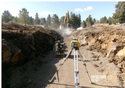
AID MCPH2 - Sta 764+50 54-IN ID profile wall HDPE pipe, placement and grading of pipe bedding mtrl 04-03-25
