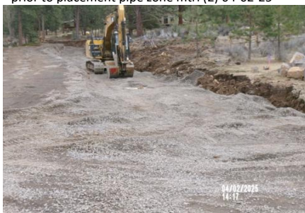
AID MCPH2 - Sta 791+50 54-IN ID profile wall HDPE pipe, 0.75-IN - 0 Aggregate Type A trench backfill in pipe zone 04-02-25
