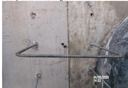
AID MCPH2 Seg2 - Sta. 718+00 Intake Structure, pipe collar, #4 dowels set in anchoring adhesive (2) 04-01-25
