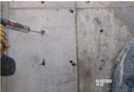
AID MCPH2 Seg2 - Sta. 718+00 Intake Structure, pipe collar, application of Simpson AT-3G hybrid acrylic anchoring adhesive 04-01-25
