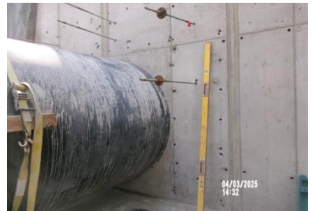
AID MCPH2 Seg2 - Sta. 718+00 Intake Structure, pipe collar adhesive dowel layout + drilled holes 04-01-25
