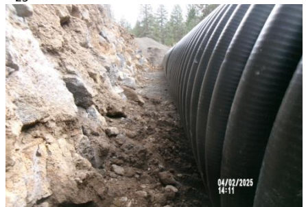
AID MCPH2 - Sta 788+75 54-IN ID profile wall HDPE pipe, rock slough removed from pipe zone prior to placement pipe zone mtrl (1) 04-02-25
