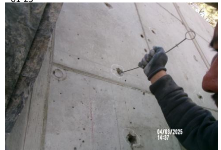
AID MCPH2 Seg2 - Sta. 718+00 Intake Structure, pipe collar adhesive dowel drilled holes, bottle brush cleaning 04-01-25
