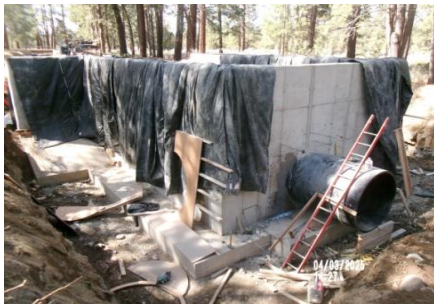
AID MCPH2 Seg2 - Sta. 718+00 Intake Structure, wall cure, plug & patch tie holes + form and bar for pipe collar 04-01-25
