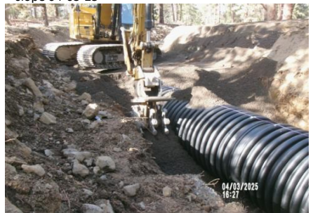
AID MCPH2 - Sta 814+00 54-IN ID profile wall HDPE pipe, initial backfill densification (2) 04-03-25
