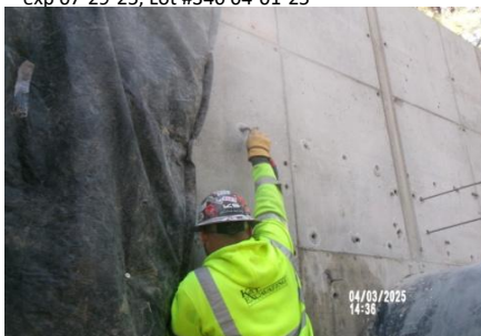
AID MCPH2 Seg2 - Sta. 718+00 Intake Structure, pipe collar adhesive dowel drilled holes, compressed air cleaning 04-01-25
