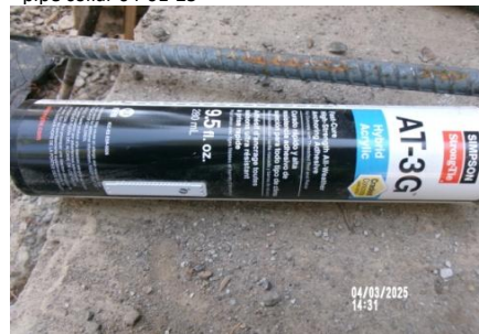
AID MCPH2 Seg2 - Sta. 718+00 Intake Structure, Simpson AT-3G hybrid acrylic anchoring adhesive 04-01-25
