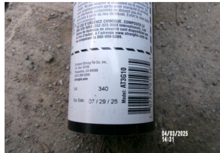
AID MCPH2 Seg2 - Sta. 718+00 Intake Structure, Simpson AT-3G hybrid acrylic anchoring adhesive, exp 07-29-25, Lot #340 04-01-25
