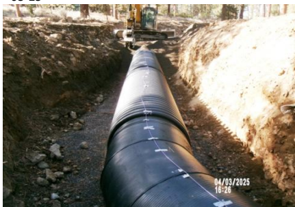
AID MCPH2 - Sta 814+00 54-IN ID profile wall HDPE pipe, initial backfill densification (1) 04-03-25
