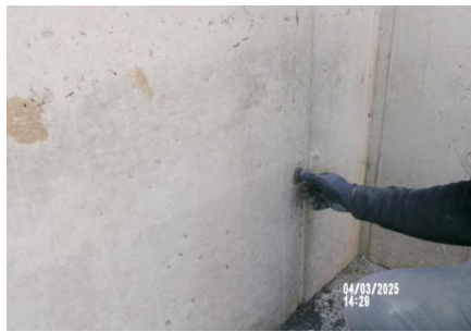
AID MCPH2 Seg2 - Sta. 718+00 Intake Structure, walls, plug and patch tie holes 04-01-25
