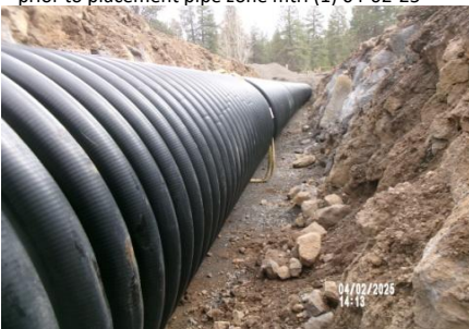
AID MCPH2 - Sta 788+75 54-IN ID profile wall HDPE pipe, rock slough removed from pipe zone prior to placement pipe zone mtrl (2) 04-02-25
