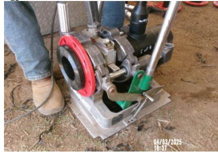
AID MCPH2 - Butt fusion welding 4-In irrigation turnout assembly pipe and fittings 04-03-25
