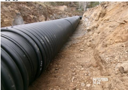
AID MCPH2 - Sta 789+75 54-IN ID profile wall HDPE pipe, rock slough removed from pipe zone prior to placement pipe zone mtrl (1) 04-02-25
