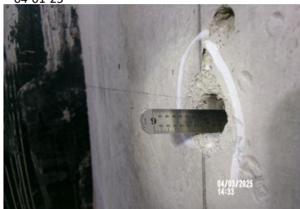
AID MCPH2 Seg2 - Sta. 718+00 Intake Structure, pipe collar adhesive dowel drilled holes 5-inches depth 04-01-25
