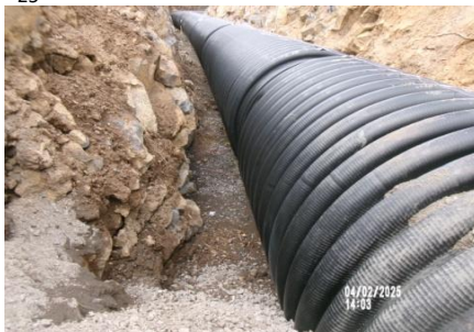
AID MCPH2 - Sta 789+75 54-IN ID profile wall HDPE pipe, rock slough removed from pipe zone prior to placement pipe zone mtrl (2) 04-02-25
