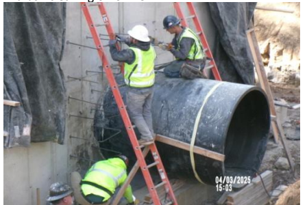
AID MCPH2 Seg2 - Sta. 718+00 Intake Structure, pipe collar, #4 dowels set in anchoring adhesive (1) 04-01-25
