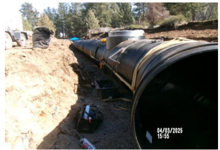
AID MCPH2 - Sta 765+50 54-IN ID profile wall HDPE pipe install and field joint fusion 04-03-25
