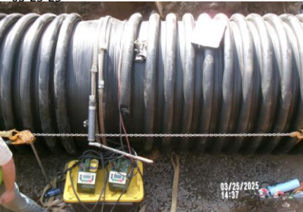
AID MCPH2 - Sta 777+90 54-IN ID profile wall HDPE pipe joint filed fusion 03-25-25
