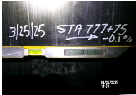
AID MCPH2 - Sta 777+75 54-IN ID profile wall HDPE pipe QA pipe slope measurement -0.1% slope 03-25-25
