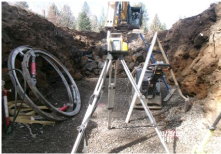
AID MCPH2 - Sta 777+20 54-IN ID profile wall HDPE pipe trench excavation and placement pipe bedding mtrl 03-25-25
