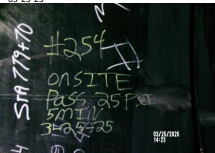
AID MCPH2 - Sta 779+70 54-IN ID profile wall HDPE pipe field joint #254 air pressure test PASS 03-25-25
