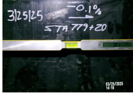
AID MCPH2 - Sta 779+20 54-IN ID profile wall HDPE pipe QA pipe slope measurement -0.1% slope 03-25-25
