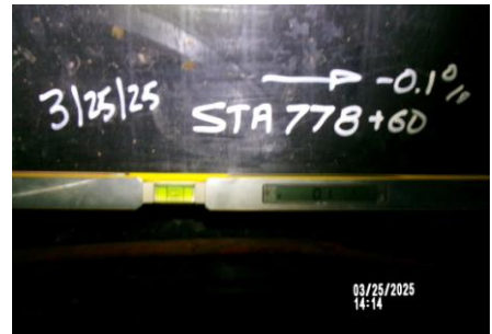
AID MCPH2 - Sta 778+60 54-IN ID profile wall HDPE pipe QA pipe slope measurement -0.1% slope 03-25-25
