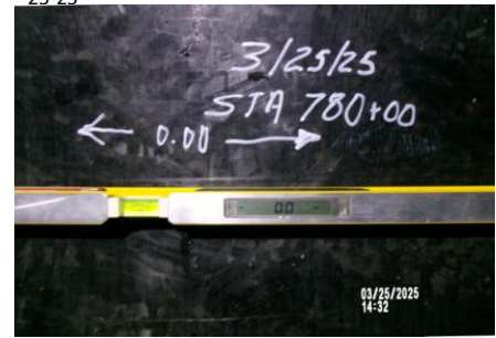
AID MCPH2 - Sta 780+00 54-IN ID profile wall HDPE pipe QA pipe slope measurement 0.0% level 03-25-25
